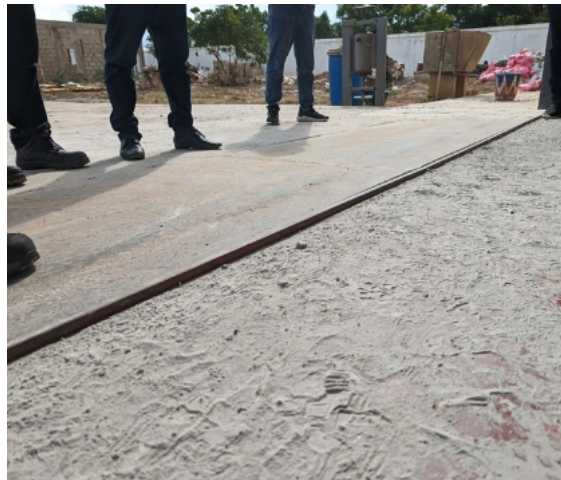
Fig 23 Unacceptable floor surface/ Stepped surface
