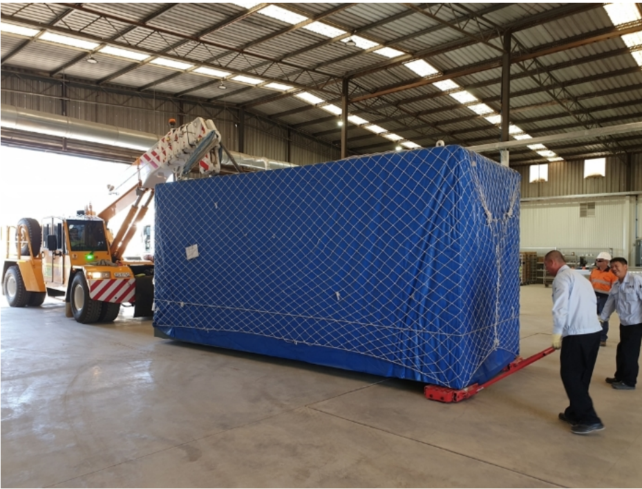
Figure 22 shows Franna lifting on end of the cabins and installation team guiding the cabin using trolleys.
