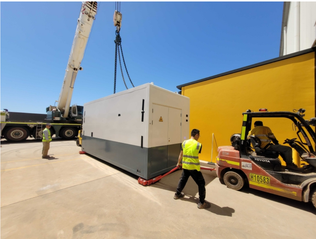
Figure 19 shows the Crane positioning the cabin onto the trolleys and the Forklift ready to move.
