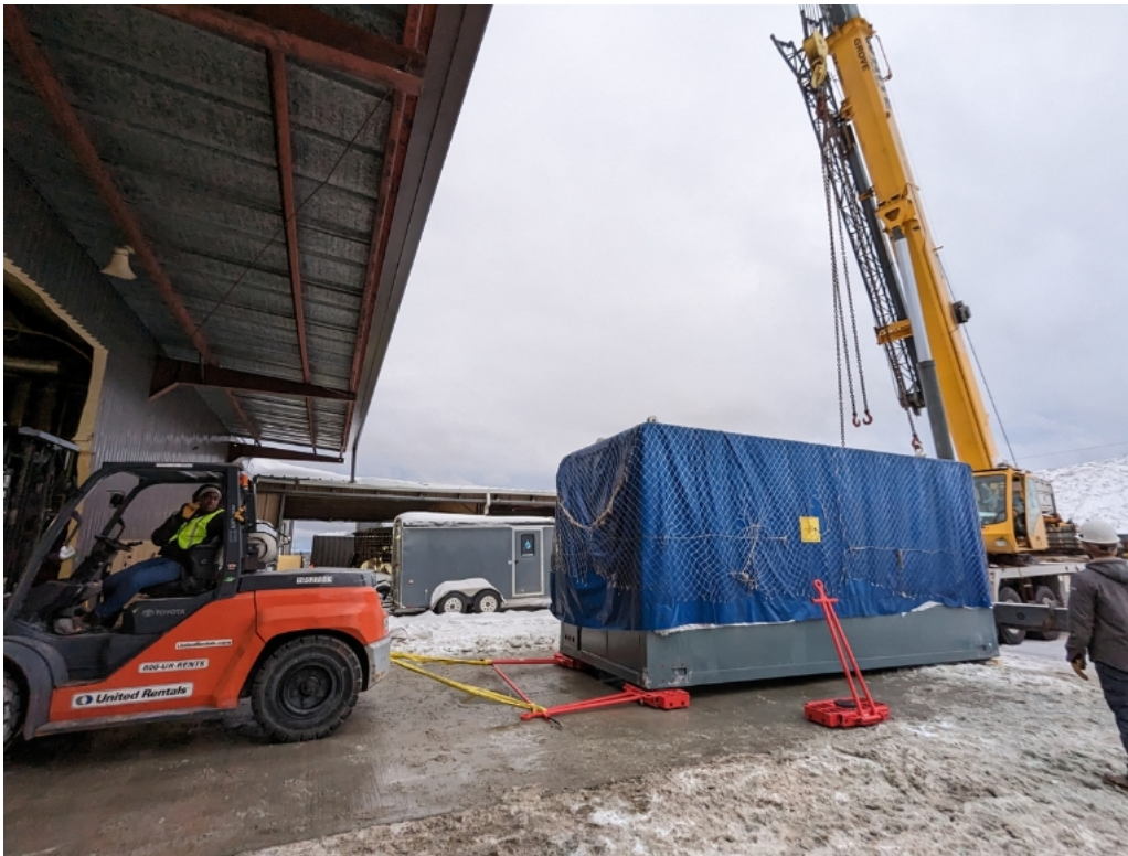
Figure 20 shows the trolleys attached to the forklift by the aid of connecting rod and slings.
