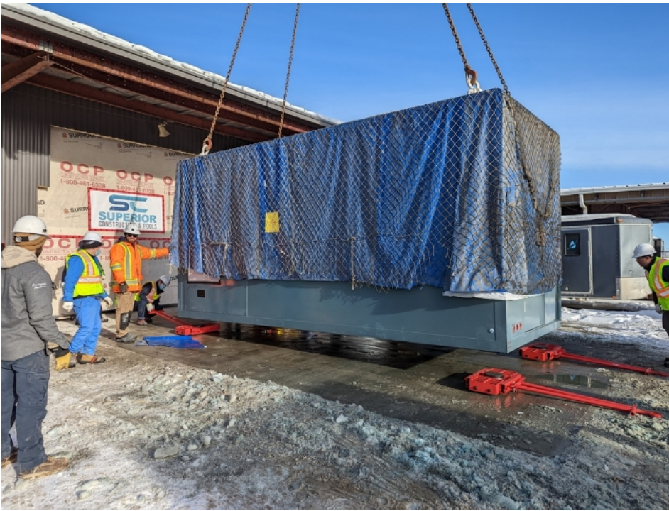
Figure 18 Unloading the cabin onto the trolleys - note the cabin is evenly balanced.
