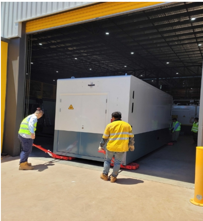
Figure 21 shows the installation team guiding the Trolleys to move the cabin inside the facility.
