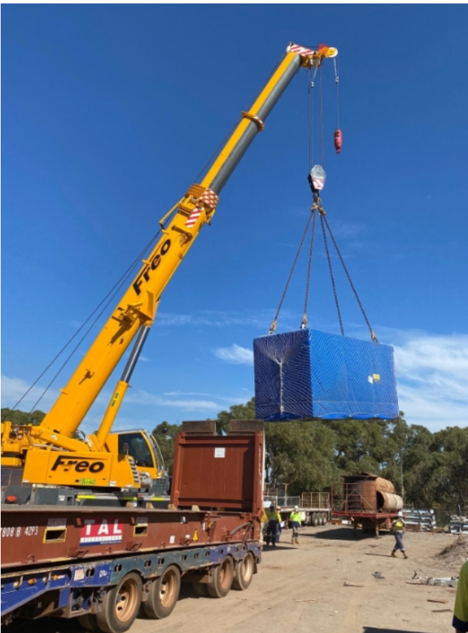
Figure 5 Image of crane lifting a cabin off the back of a truck.
