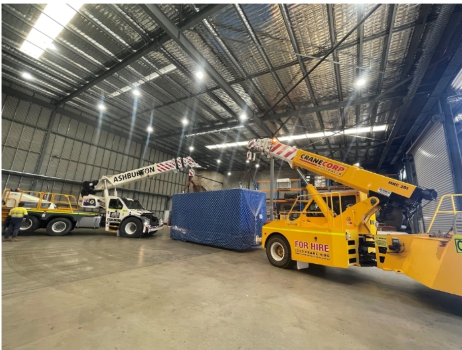
Figure 10 shows two Frannas moving the LINAC Cabin to its final position inside the facility.
