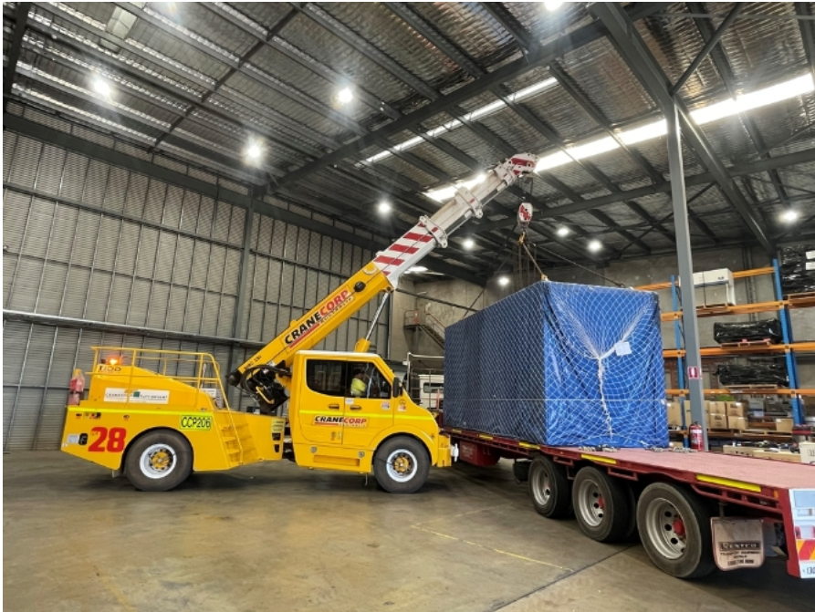
Figure 11 shows a franna unloading a Modulator Cabin from the truck inside the facility
